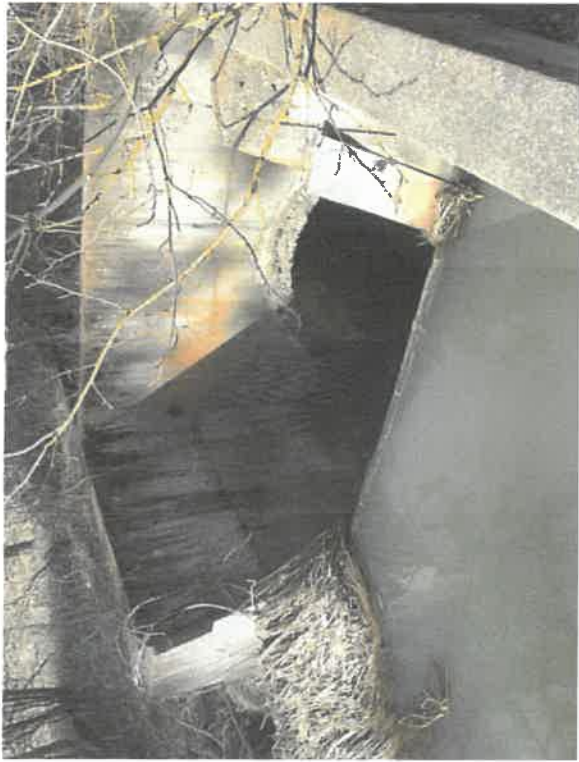
Eagle Bend Preserve Photopoint #23b: Old irrigation gate/structure along southern property boundary. Frame 2 of 2. GPS coordinates: 47.17582 -120.89038
