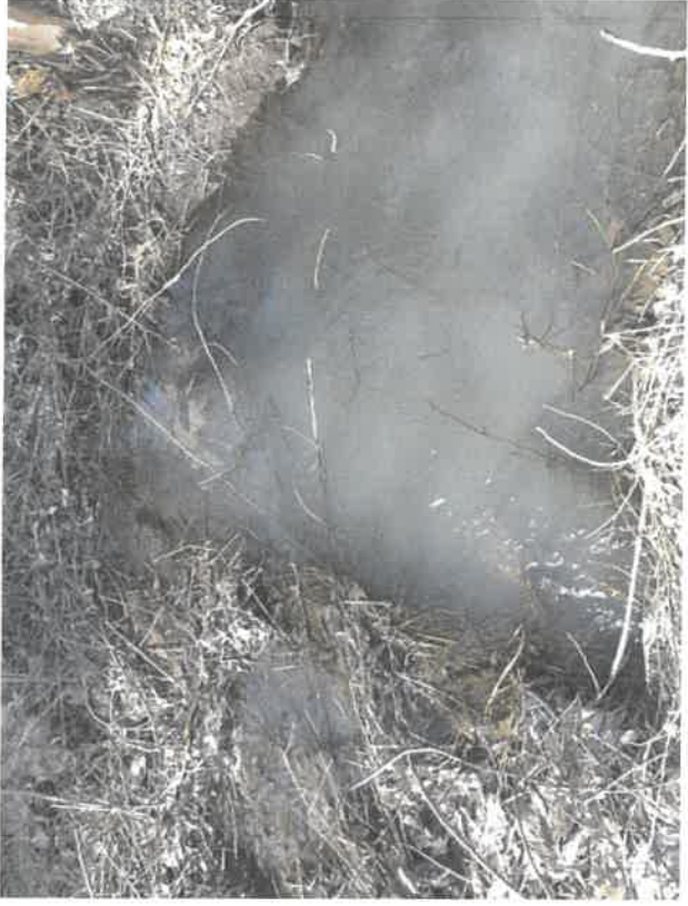
Eagle Bend Preserve Photopoint #18: Culvert under McDonald Road at southeast end of larger pond. GPS coordinates: 47.17714 -120.88927
